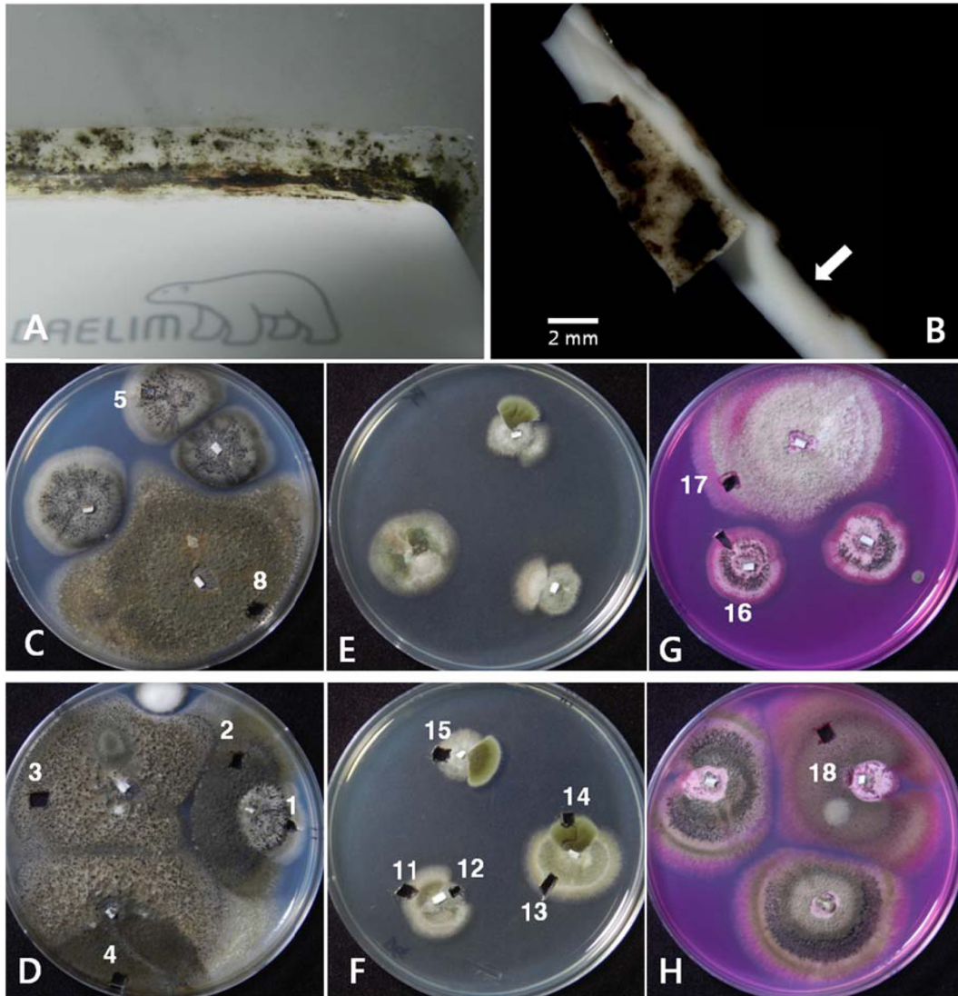
Fig. 1. Occurrence of black molds on silicon of washbasin and isolation of the fungi. A, Occurrence of black molds on silicon; B, Stereomicroscope examination of silicon blocks. White arrow indicates the fungi that grow into silicon. C-H, Isolation of fungi on various media. We isolated fungi from holes besides of numbers on plates. C, Sodium-hypochlorite untreated silicon on PDA+PS; D, Sodium-hypochlorite treated silicon on PDA+PS; E, Sodium-hypochlorite untreated silicon on DG18; F, Sodium-hypochlorite treated silicon on DG18; G, Sodium-hypochlorite untreated silicon on DRBC; H, Sodium-hypochlorite treated silicon on DRBC.
